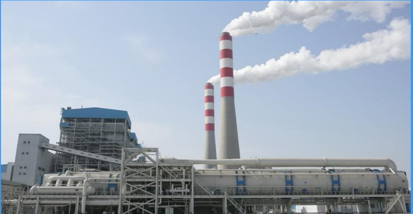
Fig.2-12 1.25 \times 10^4 \text{ m}^3/\text{d} MED Equipments build by Huanghua power plant in 2008
